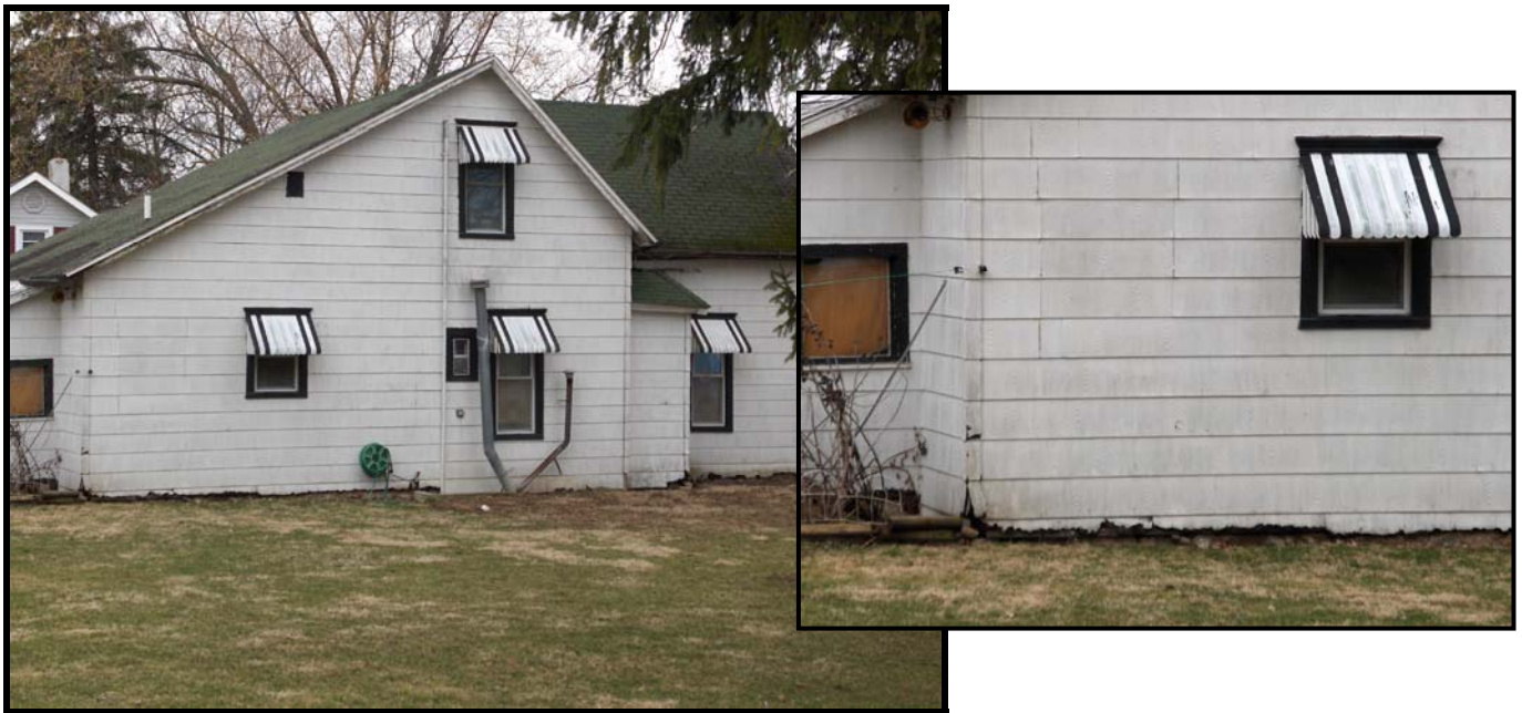
Rotting siding located along the bottom of the house 271 Main Street
