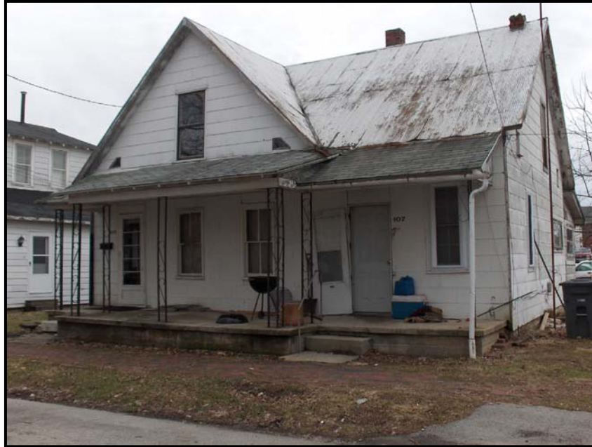
Substantial roof repair needed (105-107 Jefferson Street)
