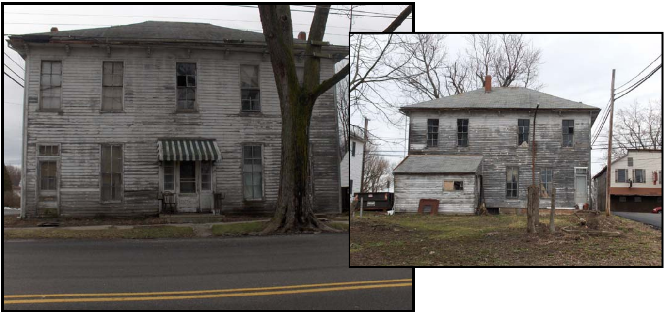
Warped and missing siding, broken windows 115 Main Street
