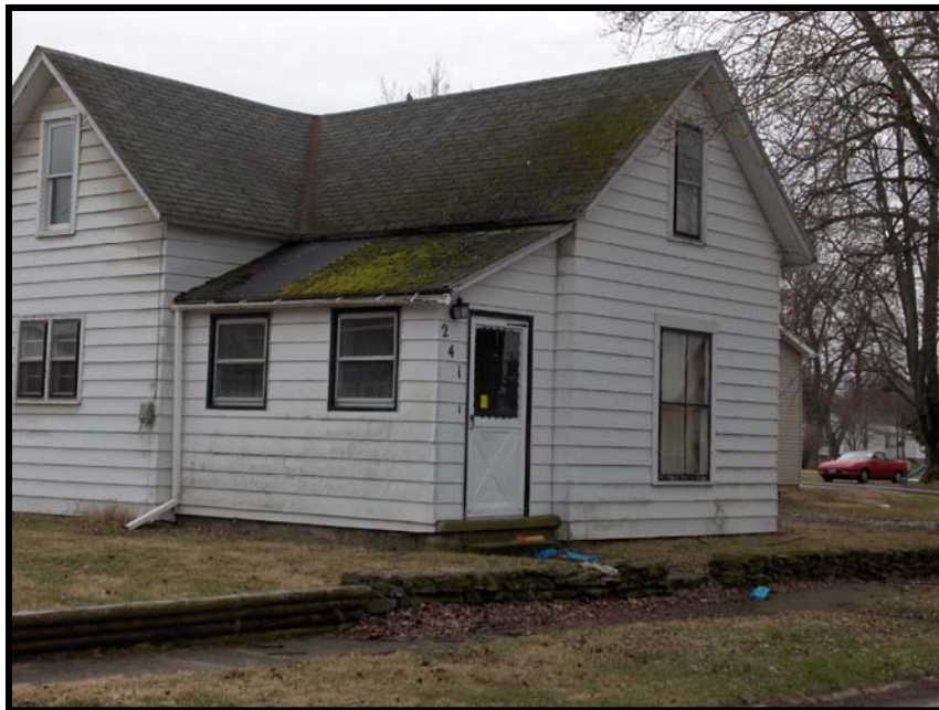
Substantial roofing and siding repair needed (the yellow sticker on the front door is a notice of foreclosure sticker) 241 Jefferson Street
