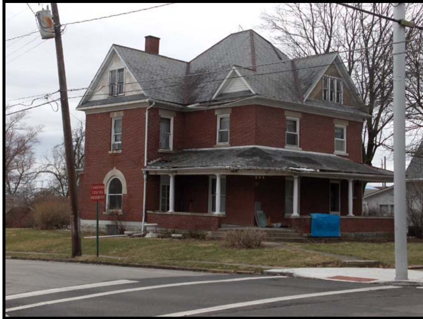
Substantial disrepair of the gutters and roof, particularly along the front porch 201 Main Street
