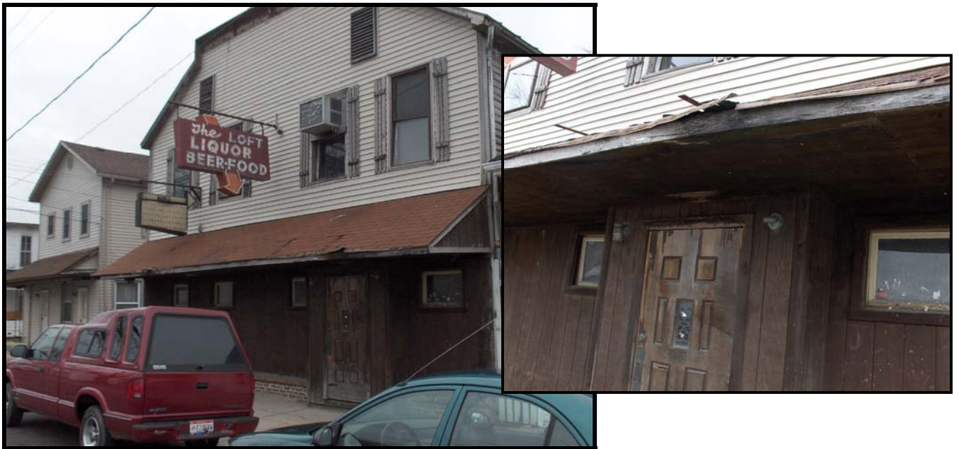
Former business site with residential apartment above, now vacant and in substantial disrepair 114 Main Street
